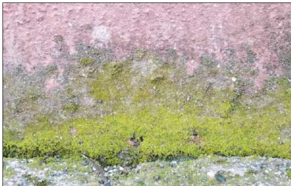
Fig 1: Green algae on the wall of the wall of the hostel
